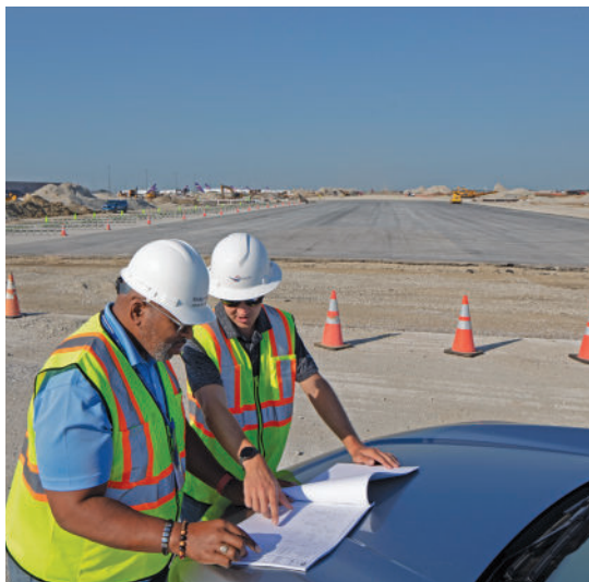
FLYING HIGH Kimley-Horn is overseeing a three-year runway reconstruction project at the Indianapolis Airport.
