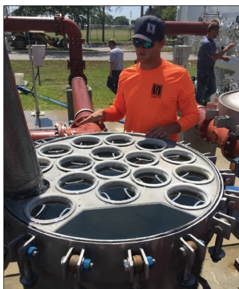
Figure 13. Bag filter vessel.
