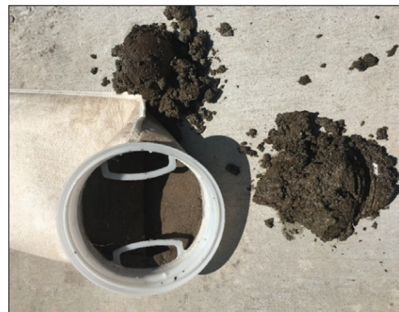
Figure 12. Sand and foulant on bag filters.
