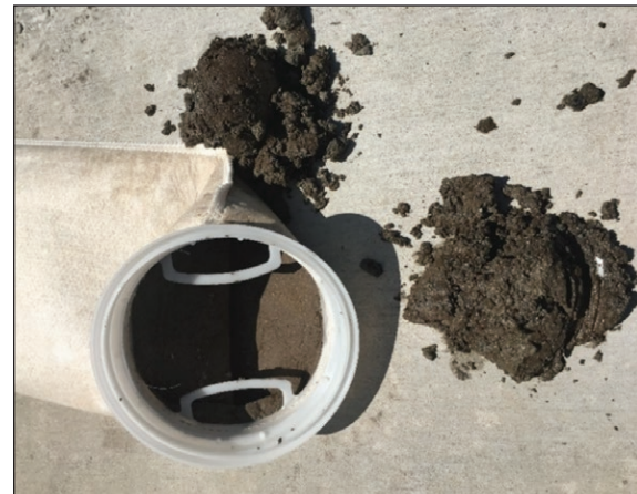
Figure 12. Sand and foulant on bag filters.
