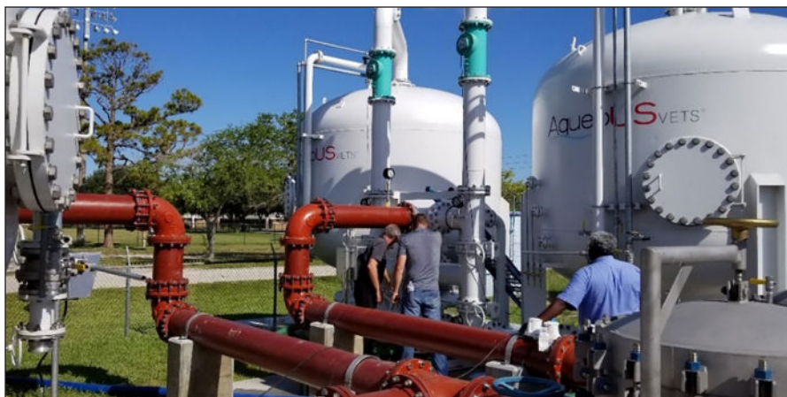
Figure 11. Start-up of the system.
