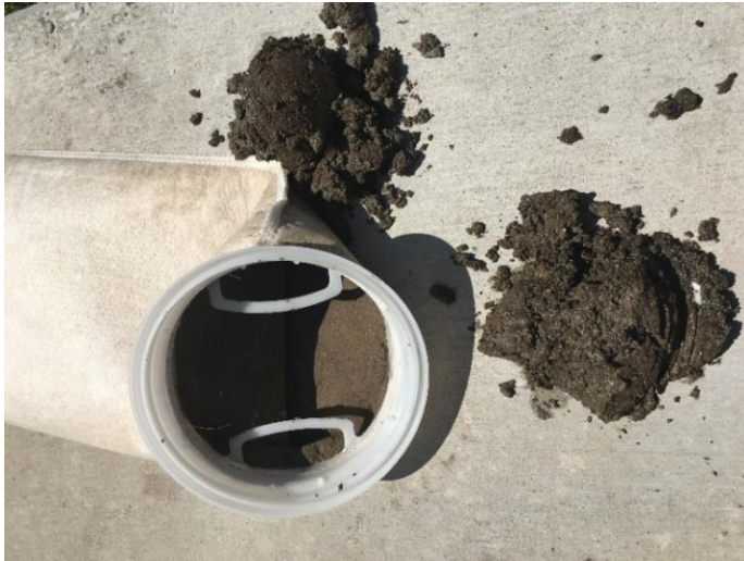
SAND & FOULANT ON BAG FILTERS
